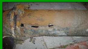
Fig. 8 Corrosion of Xinbeitou \phi 300 mm DIP pipe (Placed for 20 years and was asphalt coated from outside and leak repair has been done at the same place one year ago)
