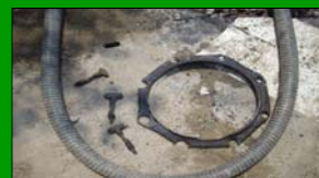
Fig. 9 Corrosion of Pressure Ring of Xinbeitou \phi 300 mm DIP (Placed for 20 years and heaviest corrosion is found at 6 o'clock direction)
