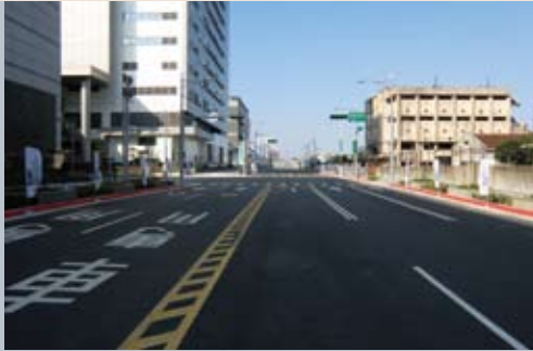
Roads are repaved as part of the underground railway project (Civil Boulevard, section B).
