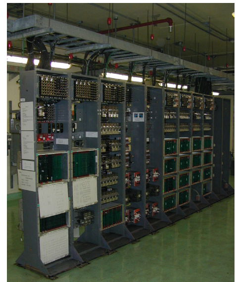
Typical Signal Equipment Room
