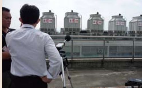
Measuring noise volume of a cooling standpipe.
